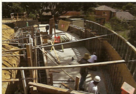
The box is then waterproofed and a condensation drain is installed in the deep end
