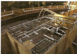
The steel and plumbing for the pool, spa, and perimeter are completed after the upper pool forms are installed
