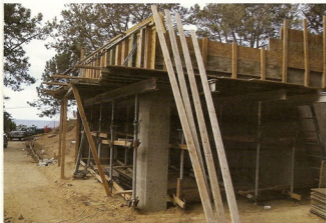
The structural box that will support the pool and spa is installed. The top of the box is approximately 2 in. (50 mm) lower than the top of the pool finish elevation
